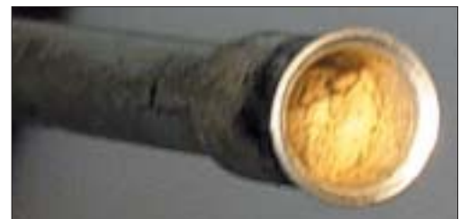
End view of an evaporator neck shows why there was no cooling. The evaporator is plugged with hardened sealer.
