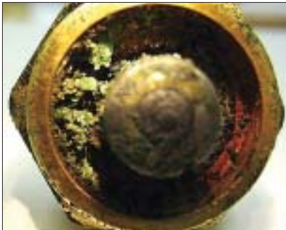
End view of solenoid valve from a recovery/recycling machine shows plugging with hardened sealer.
