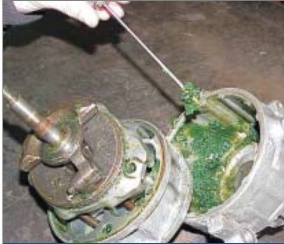
Internal compressor contamination.
